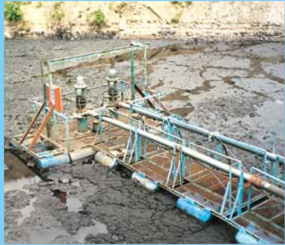
Courtesy of: Service Pump & Supply / Huntington, WV
